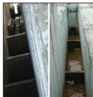
Inner view of fish pass at Naraj barrage
